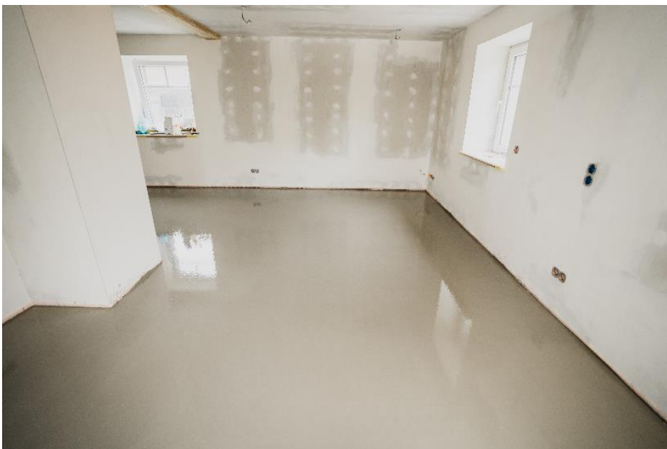
Ready for laying the vinyl floor after a short drying time: PCI Periplan Extra is suitable under textile and elastic floor coverings, is dust-reduced and very low in emissions according to GEV-EMICODE EC 1 PLUS.. (© PCI Augsburg GmbH, Link to high-resolution photo)
