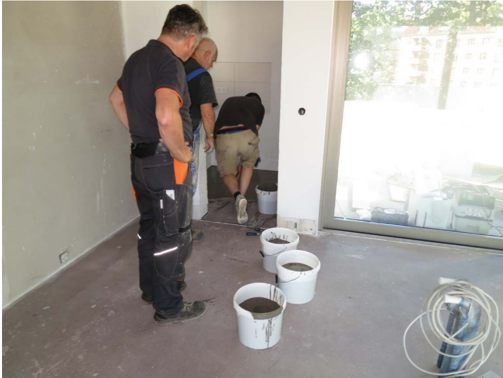
Fig. 6: Client and builder in one: Holger Andreas installed the floor himself and opted for self-levelling PCI Periplan Multi levelling compound.
